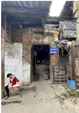
墙体歪散、坍塌
